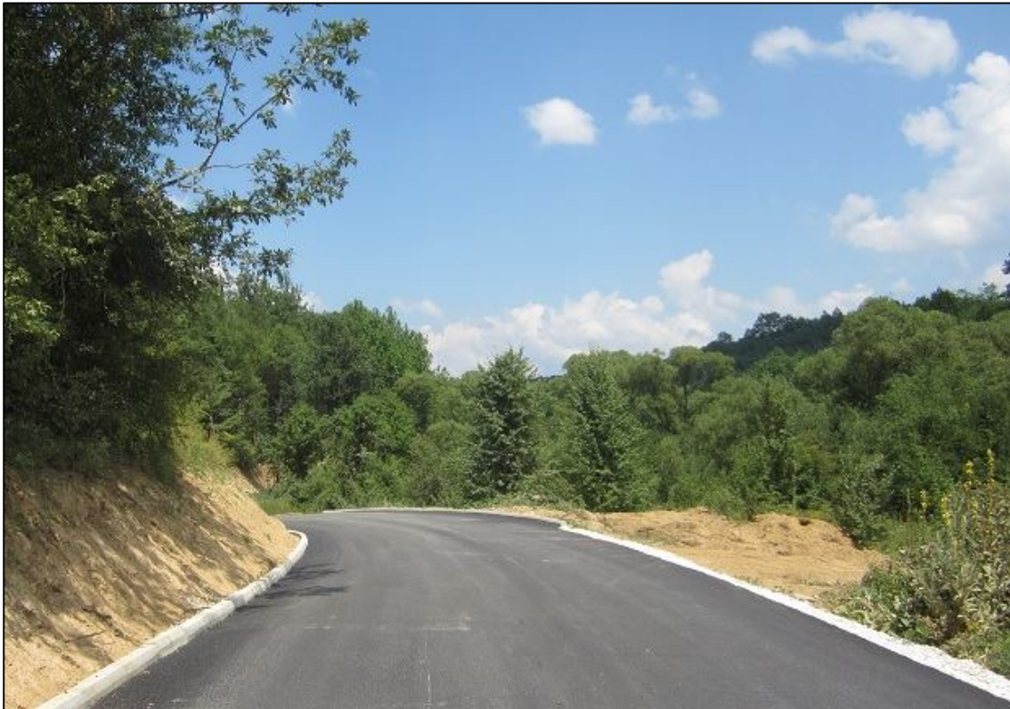
The reconstructed road connects the border area of Palja with the international route M1.13
